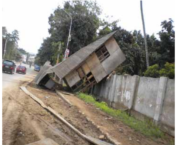
House in Cagayan de Oro leaning on a concrete wall
